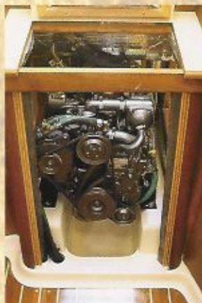
Access to the 27 horsepower freshwater-cooled Yanmar is excellent on all four sides. The insulation will keep it quiet and cool.
